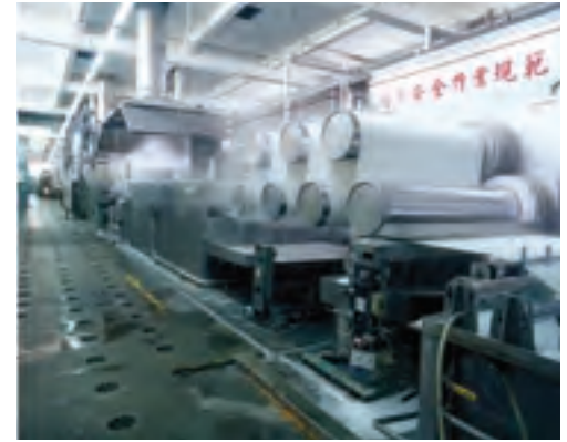
Automated Fiber Line for Staple Fiber
